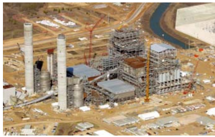
Oak Grove Power Plant Robertson County, Texas
