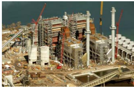
Sandow Power Plant Unit 5 Rockdale, Texas
